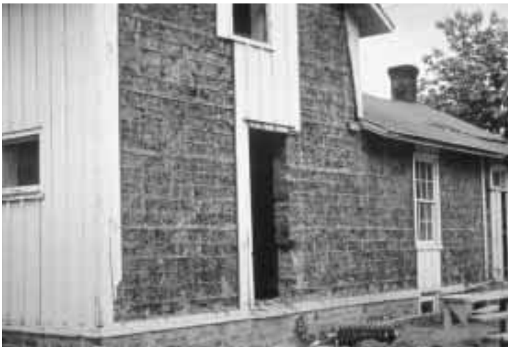
When it was demolished in the 1970s, this board-and-batten sided building in Geneva was found to be load bearing mud brick construction, originally sided with wood. Photo by David Brumberg.
