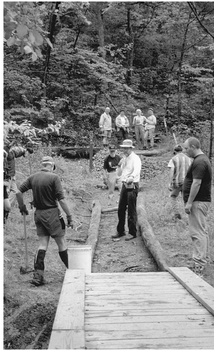
Building a greenway in Georgia's Amicalola Falls State Park off the Appalachian Trail.
